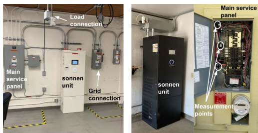
Figure 7: Photos of installed sonnen units. Left is the lab setup while right shows the home setups.
